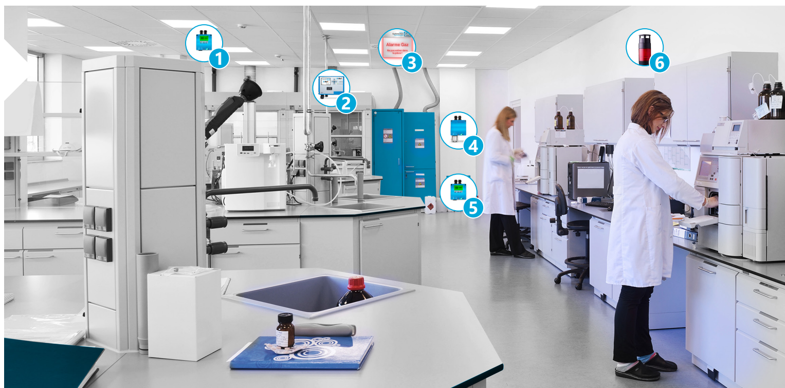
1 Hydrogen transmitter CH 4 2 D-ReX (PoS) 3 Warning panel 4 Oxygen transmitter 5 CO 2 transmitter 6 Visual alarm
